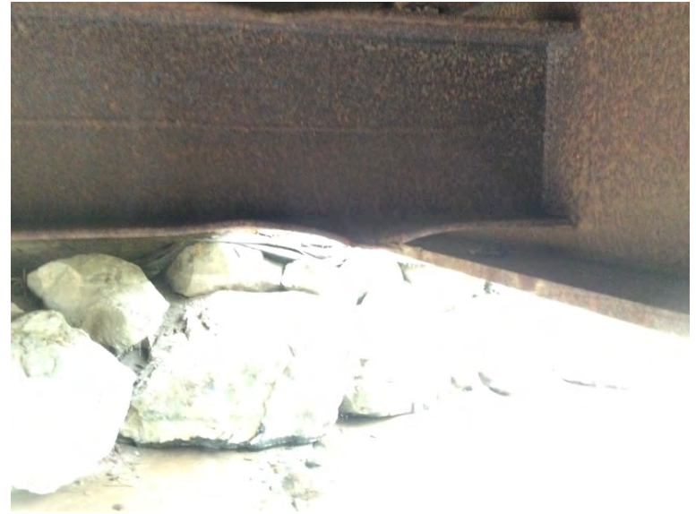
Minor damage to center span bracing
